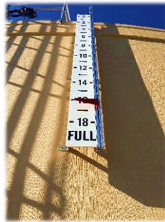
New tank's depth gauge
